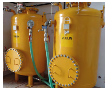
Pump & Treat Anlage
